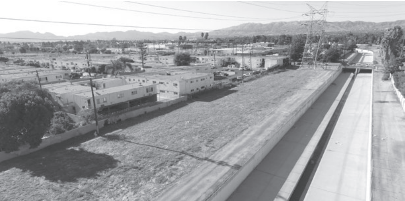
View looking north along Aliso Canyon Wash just south of Napa Street
